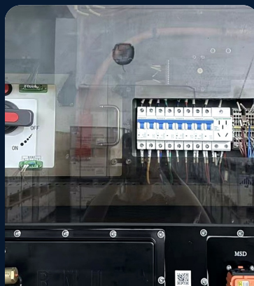
BMS / high-voltage control
